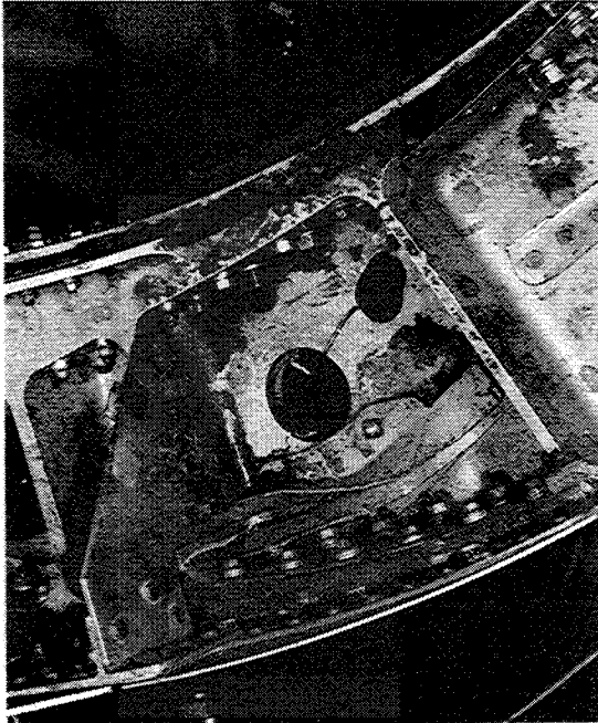
Fig. 13 Final failure at the fuel pipe holes.
